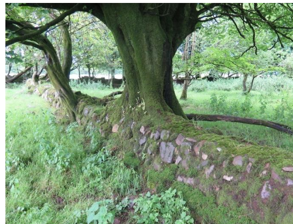
Figure 15-36: Mature trees growing from wall at Cappagh deserted farmstead
